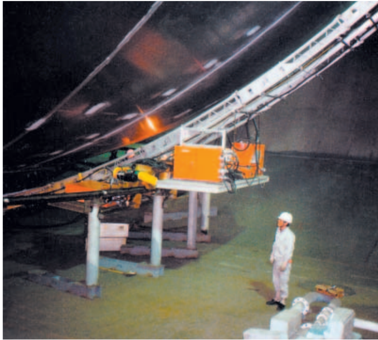
Steel boom assembly used to apply insulation for liquid natural gas storage tanks on seagoing ships. The 78 ft. lower hemisphere boom (shown above) is fitted to the 133 ft. diameter storage tank. The boom assembly was designed and analysis provided for TI Marine Contracting, AS of Norway.
